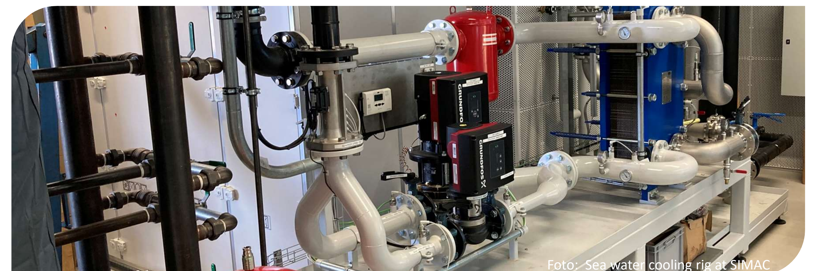
Foto: Sea water cooling rig at SIMAC
